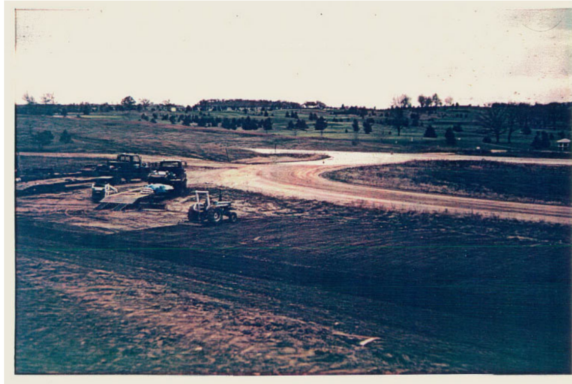
Landfill entrance looking south towards the Yahara Hills Golf Course during the first phase of construction in 1985.
